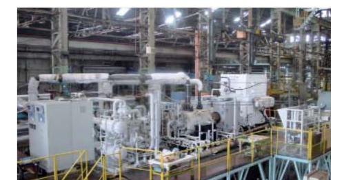
String test of electric motor driven compressor train
