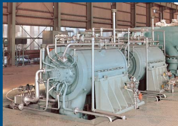
Tandem arranged steam turbine driven compressors for ammonia gas service, Ube Ammonia (Japan)
