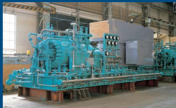
Motor driven compressor for syn. gas service, RCF (India)
