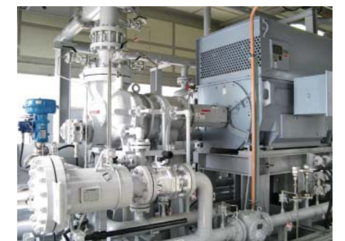
Shop Fuel gas compressor for GT drives
