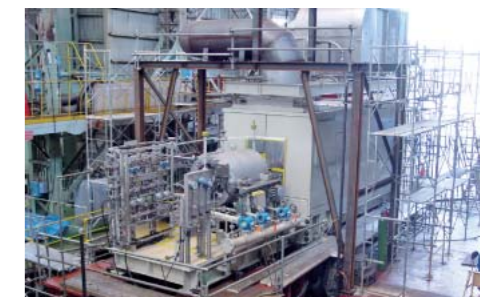
String test of gas turbine driven compressor train
