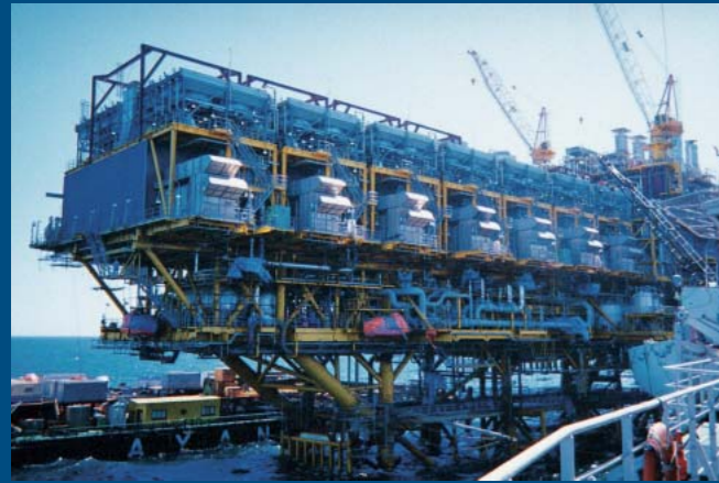
7-Compressor modules installed on SHG platform, ONGC (India)
