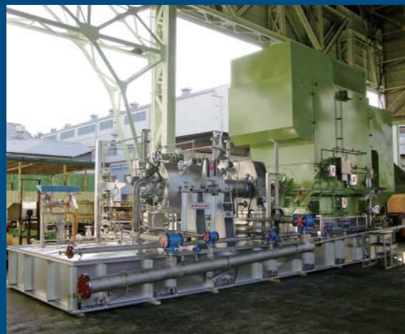
Motor driven compressor for natural gas service, Saudi Aramco (Saudi Arabia)
