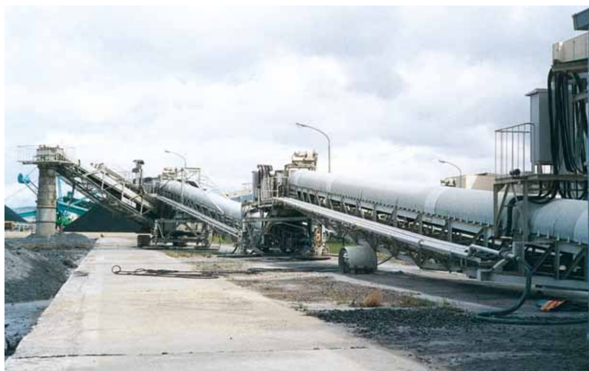
300 T/H ash disposal conveyor
