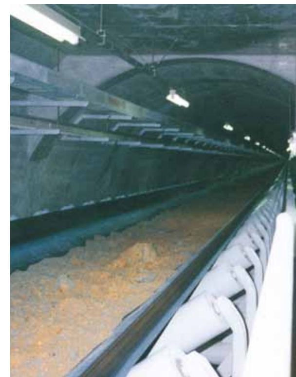
9,000 T/H belt conveyor
