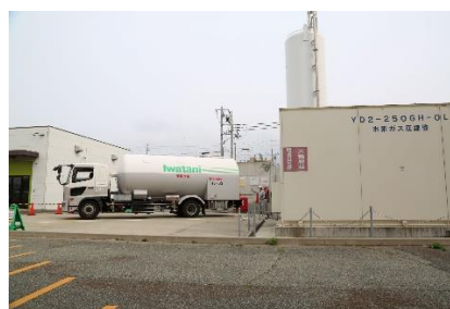
Filling a storage tank with hydrogen at the demonstration site
