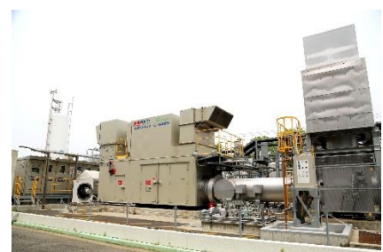
Hydrogen Power Generation Plant
