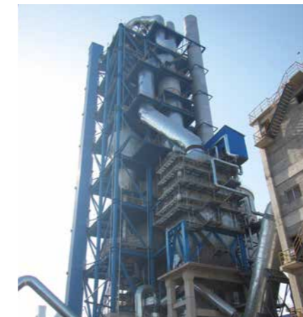
First VEGA boiler, installed at the Huaibei Zhongbei Cement plant in China
