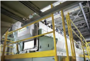
Hydrogen 30% co-firing gas engine
