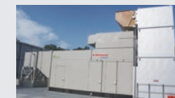
Emergency power generator
