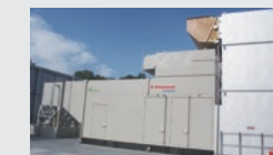
Emergency power generator
