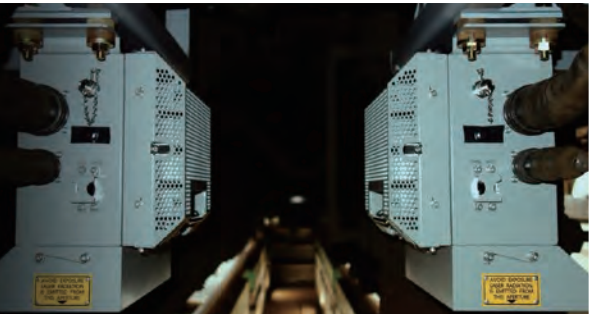
Remote track monitoring system
