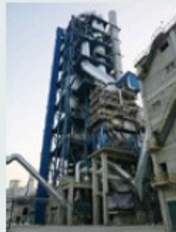
Cement plant waste heat power genera- tion facilities
