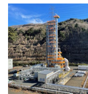
Demonstration facility in Maizuru Power Station, The Kansai Electric Power Co., Inc.
