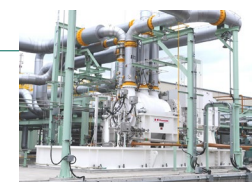
Demonstration facility of Centrifugal hydrogen compressor
