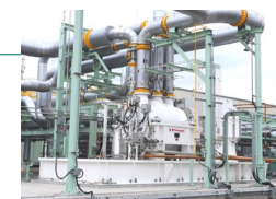
Demonstration facility of Centrifugal hydrogen compressor
