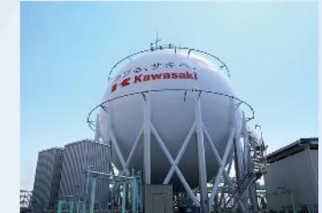
Liquid hydrogen storage tanks
