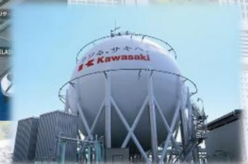
Liquid hydrogen tank
