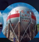
Long term storage of liquefied hydrogen
