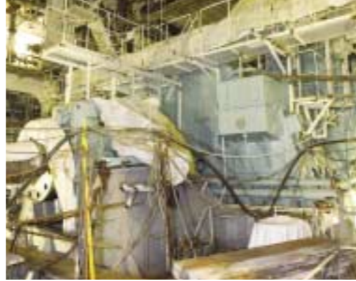
The Kawasaki URA Turbine Plant installed inside the vessel's engine room.
