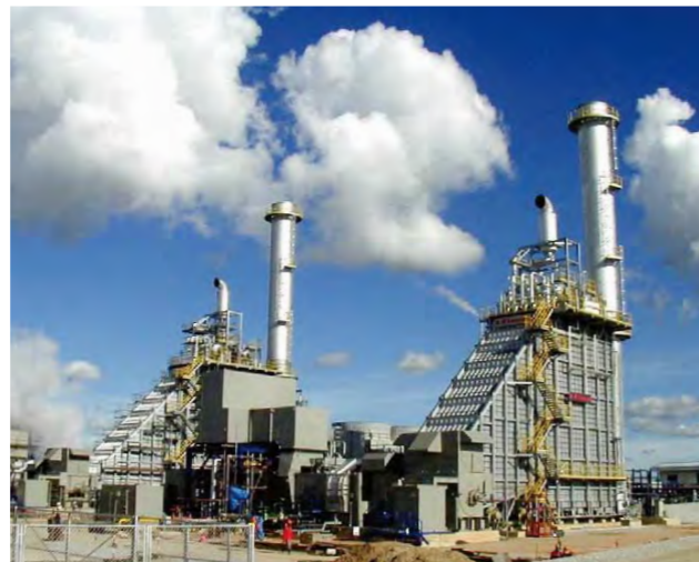
Example of the introduction of a combined cycle power generation system (TNP in Thailand, 114 MW)
