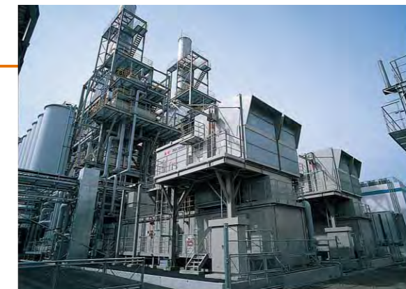
Example of installation to a food manufacturing complex
