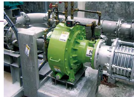
Example of installation at the Masaki Dam (Tokushima prefecture)
