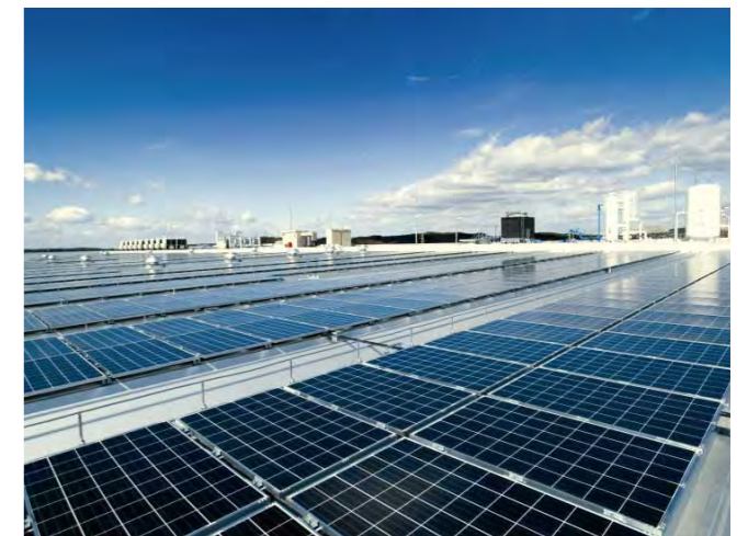
Location: West-Kobe Plant of Kawasaki Heavy Industries Capacity: 200 kW Start of operation: February 2009
