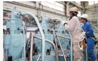
Shop test of critical equipment
