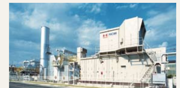
Gas turbine generation system at Akashi Works
