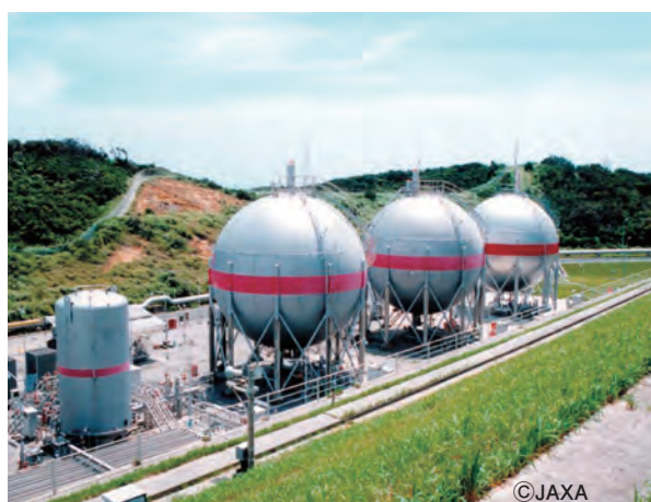
Fig.4 Japan's largest LH 2 tank
